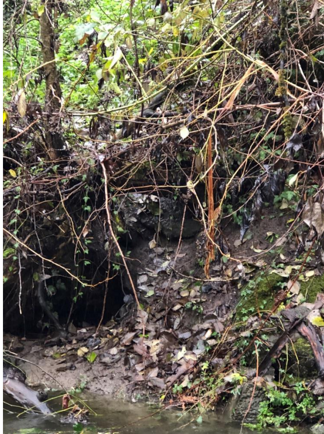
Figure 2-15: Signs of erosion downstream of I-405
